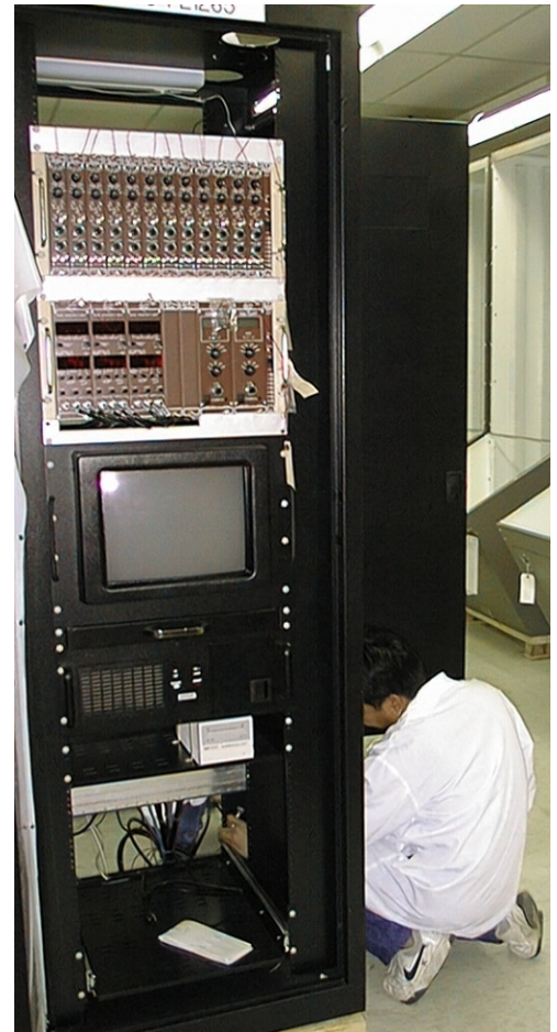
Cabinet for Programmable Logic Controllers and industrial type computer under construction
